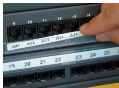
Punch block & patch panel labels
